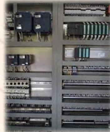
Control With S7-300 PLC
