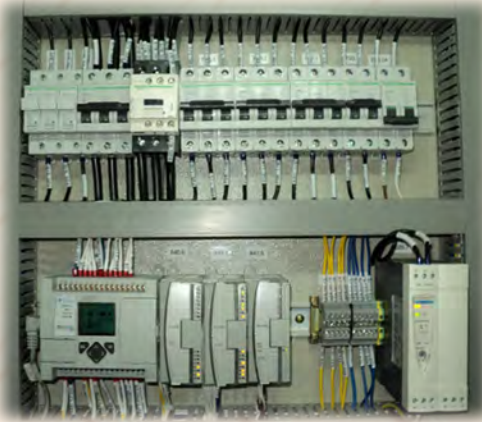
Control With AB PLC
