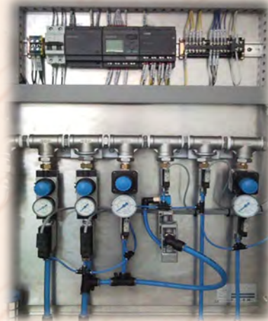
Electrical with Pneumatic Control
